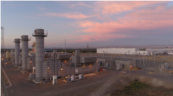
Almond 2 Power Plant.
