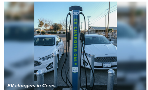
EV chargers in Ceres.
